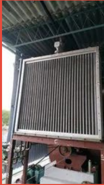
Thermic Oil Radiators
